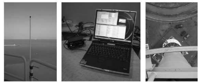
Figure 4: VHF antenna attached to a tower and AIS Receiver
